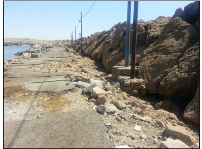
Figure 3. Damaged in Ramin Port breakwaters resulted by wave overtopping during Gonu Cyclone
