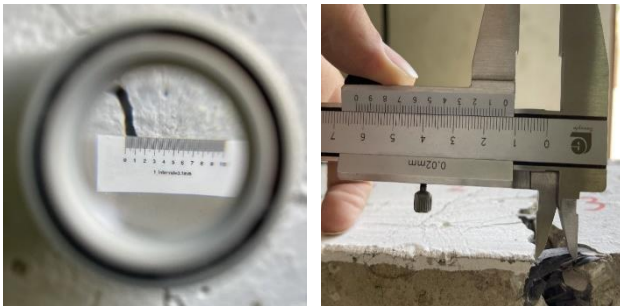
Figure 33. Measurement of the crack dimensions
